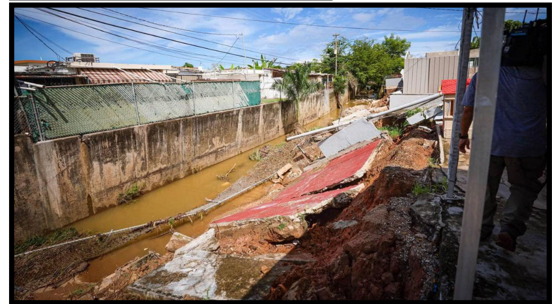
Figure 4 and 5: Images of existing condition and repairs performed by MSJ due to impacts from 27 October 2023 rain event.
